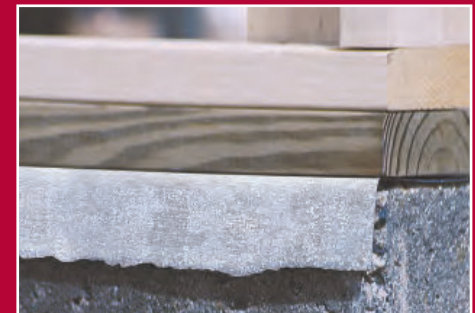
ACQ treatment corrodes aluminum flashing
