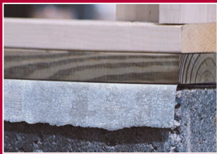
ACQ treatment corrodes aluminum flashing
